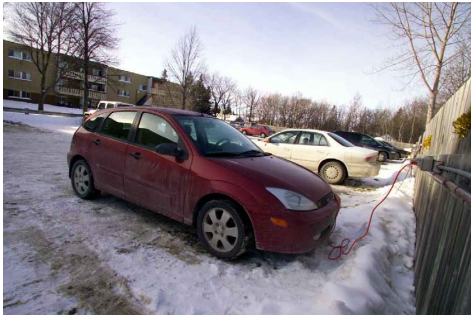
More than 60 parking lot controllers were installed at Charlesdale Gardens in Winnipeg to help reduce operating costs for Globe General Agencies.
